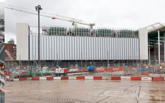
T2A cooling station
